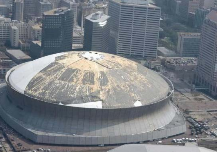
Traditional Roof System after Katrina (Louisiana Superdome)
